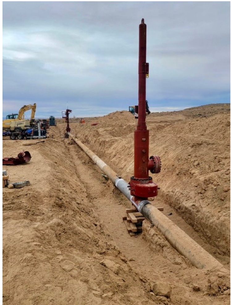
Running Horse Pipeline is continuing to repair and replace pipeline sections and install stopple plugs both upstream and downstream of the isolated pipeline section.
